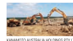
KANAMOTO AUSTRALIA HOLDINGS PTY LTD
