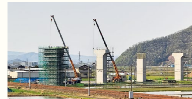
北陸新幹線の高架工事 Construction of an Elevated Structure for the Hokuriku Shinkansen
